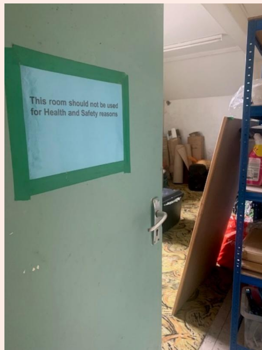
Storeroom access restriction
